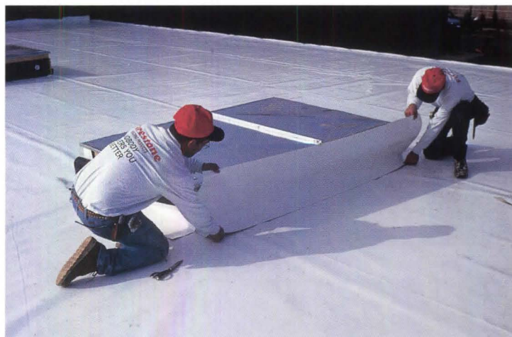
Narrow rolls of TPO are labor intensive to install, but are more stable.
