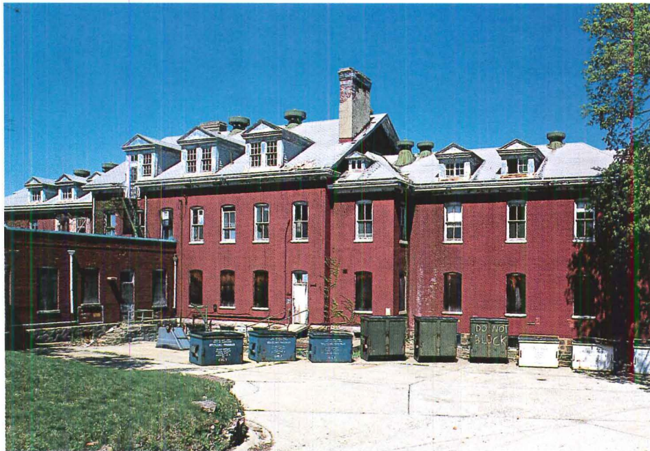
Abandoned for over 25 years and now in a state of decay, the original 1911 army hospital in Queens is slated for rehabilitation and adaptive reuse as classrooms for the FDNY's new training facility.
