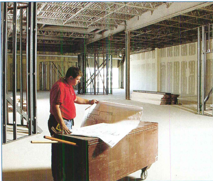
Skip Pastore, site manager for Barrier Corp., reviews construction plans following application of the gypsum concrete underlayment floor. The floor is ready for continued trade traffic within 24 hours.
