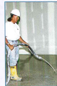
The gypsum underlayment mix was pumped via hoses and poured directly onto the floor.
