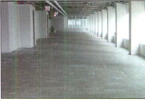
The existing concrete floors in this renovated 26-story office building in downtown Philadelphia were cracked and uneven.
