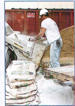
Bags of gypsum concrete underlayment were mixed with sand and water to create a slurry.
