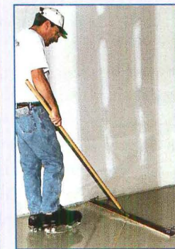
The underlayment was screeded to the thickness of the elevation pins to achieve a smooth, even surface.
