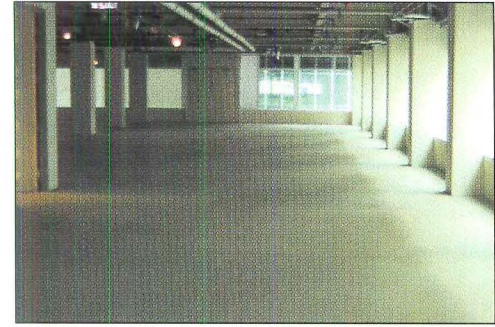
The new gypsum concrete underlayment provides a smooth, even surface, ready for floor finish material installation. The entire application was completed for less than half the cost of using a portland cement-based product.
