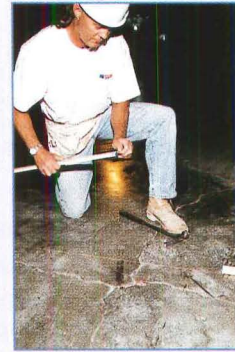
The existing concrete and terrazzo floors in the 18,500-sq.-ft. retail location space were cracked and uneven.
