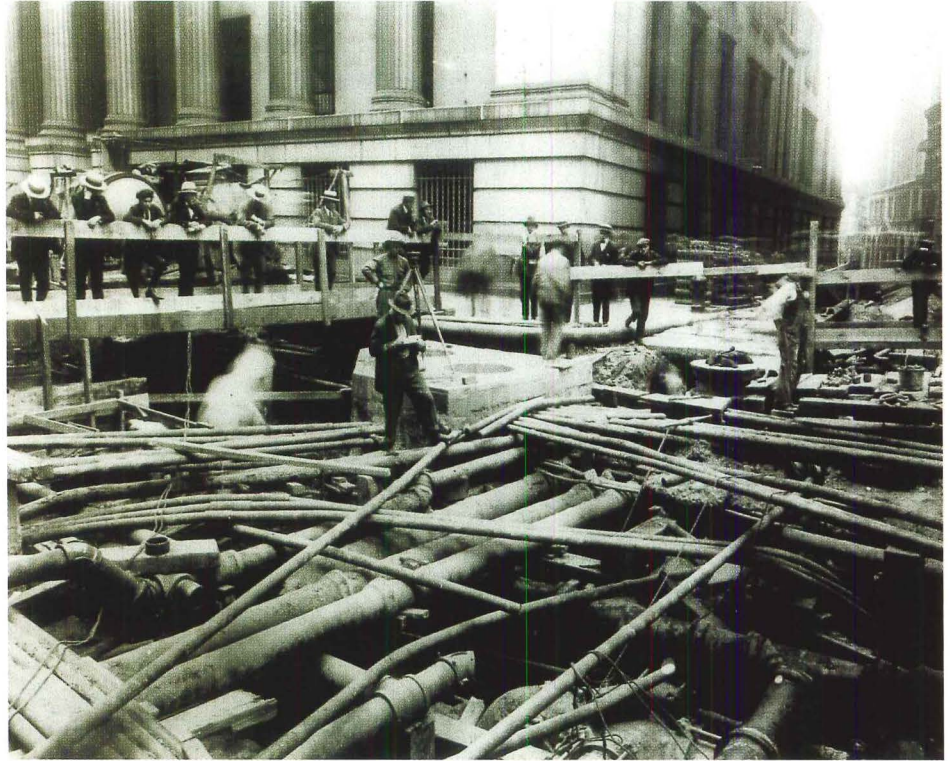
Peeling back the street surface of Lower Manhattan in 1913 revealed a tangled web of pipes and ducts, much of which is still part of New York City's complex infrastructure, and has been for over 100 years.
