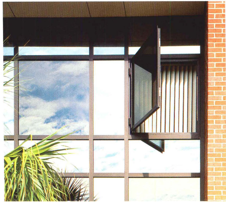
Fixed and movable features such as vertical blinds shown above can block and reflect direct sunlight entering through windows.
