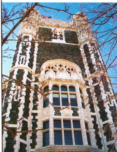
A New York City landmark gets a facelift with a new material (168).
