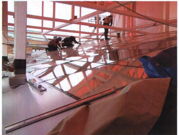
Workers replace the Wexner's skylight with a highly engineered triple-glazed system (above). The construction called for maneuvering around Eisenman's scaffoldinglike facade (top).
