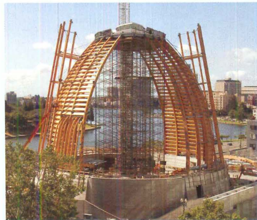
The cathedral structure has inner and outer shells of vertical glue-laminated ribs (left). The inner one, made from curved ribs, takes its shape from the surfaces of a pair of intersecting spheres, while the outer shell is composed of straight elements that define segments of two cones.
