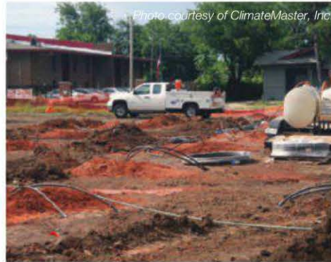
For the United Way's headquarters for Central Oklahoma, a geothermal system was installed with 25 wells located beneath the new parking lot.
