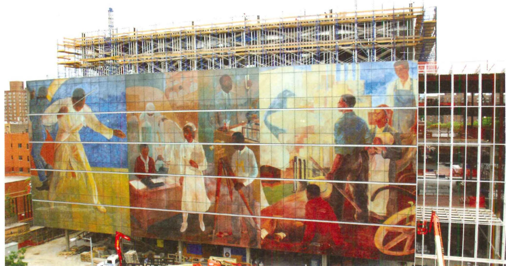
The curtain wall facade on the Harlem Hospital New Patient Pavilion features a digitally applied artistic mural that provides light control while still allowing vision out.
