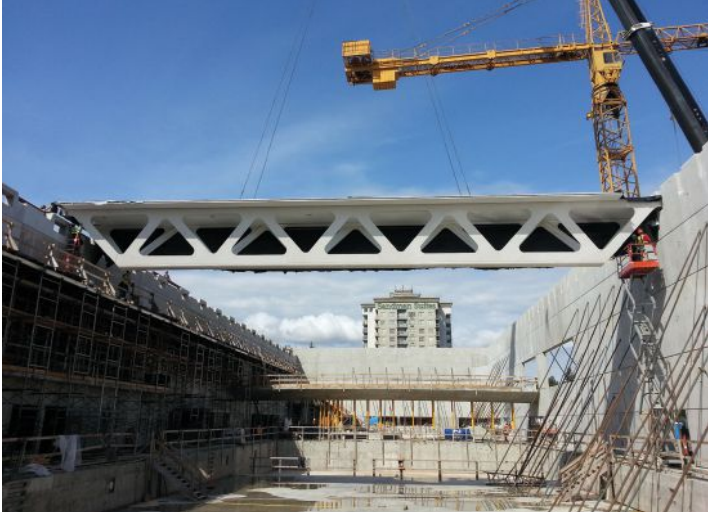
PREFABRICATED, V-SHAPED WOOD TRUSSES ARE LOWERED INTO PLACE AT THE GUILDFORD AQUATIC CENTRE IN SURREY, BRITISH COLUMBIA.
