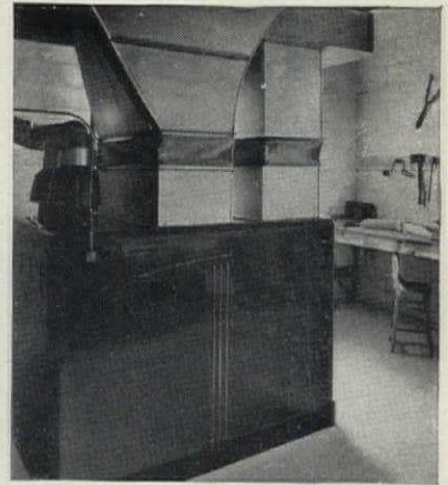
In one corner of the carpentry-workroom in the Sutton basement, stands this gleaming G-E air-conditioning and heating unit. It has turned in a 100% performance since its installation.
