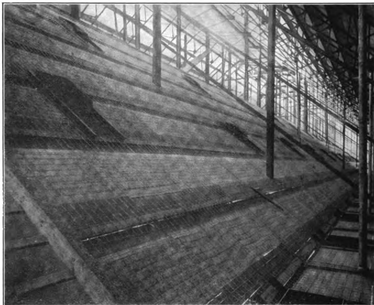
WIRE CLOTH IN PLACE READY FOR THE CONCRETE Interior of Government Coal Pockets, Bradford, R. I. Clinton Wire Cloth Co.
