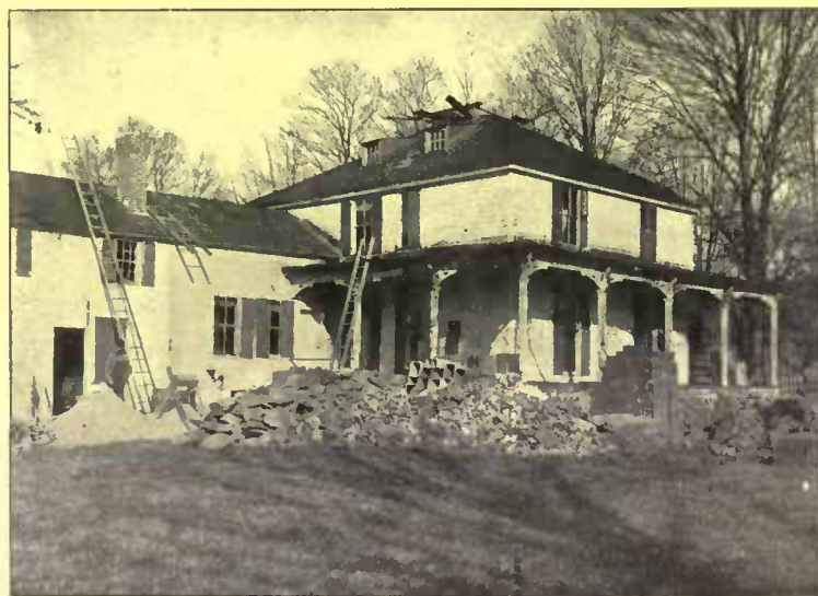
The house as it was found and in the first stages of alteration of the chimney and the dining-room
