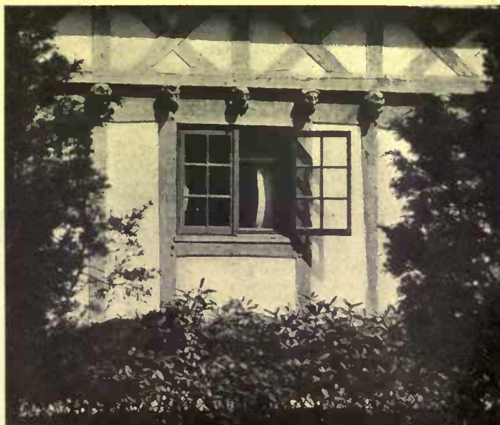
The simplest form of casement opens outward and has a stop molding, which keeps out rain and moisture
