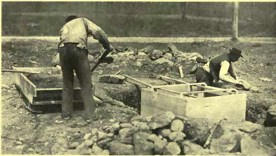
The construction is simple. A wooden "mold" is made, into which the cement is poured and allowed to harden
