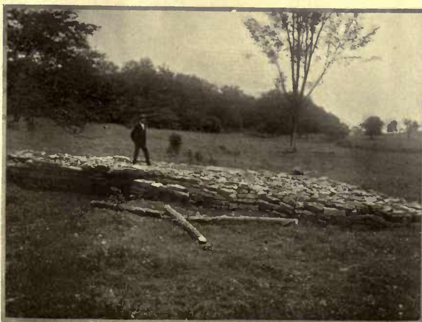
At this juncture the road bed was ready for the dirt, which was laid on a foot thick—a costly item in the bill
