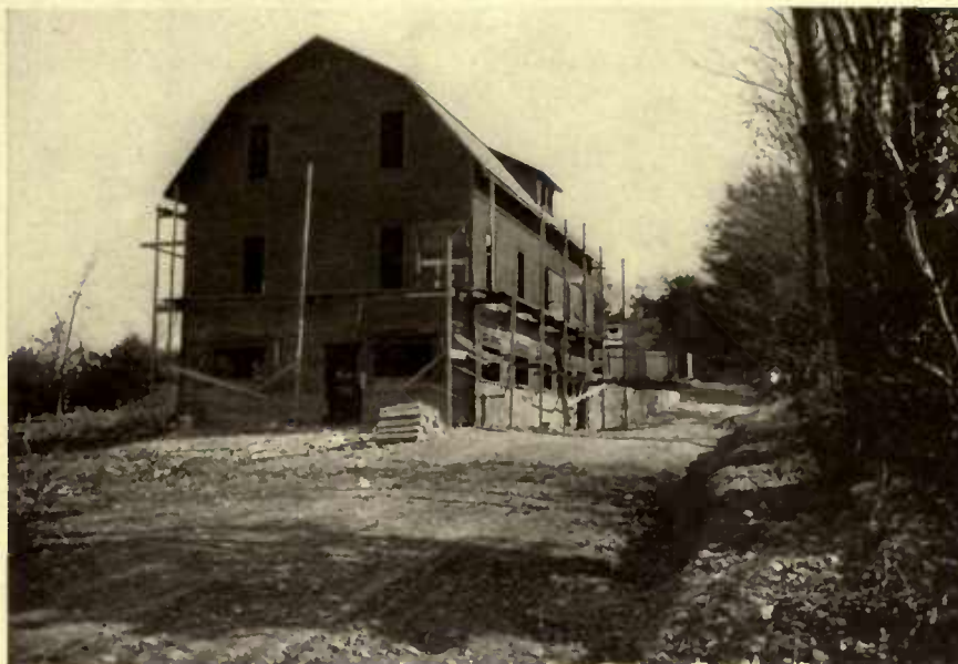
It was a cross between a city stable and a country barn. The first floor is for the horses and cows, second for carriages and wagons and the third a hay loft. Cost complete, $3,264.96
