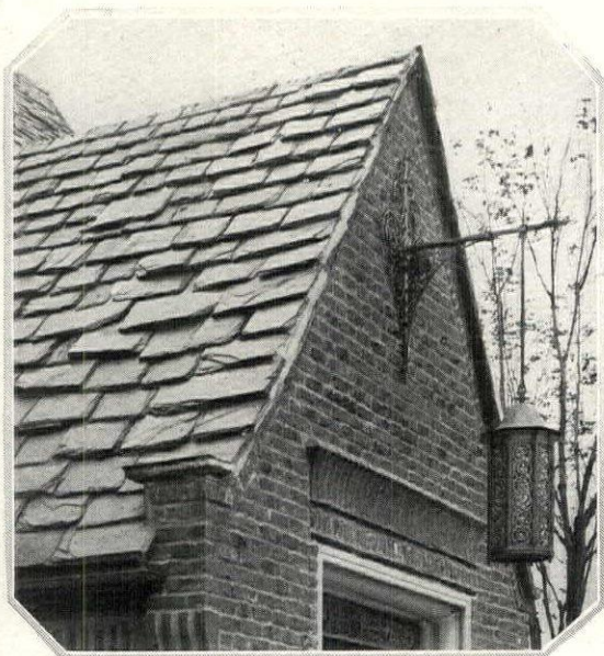
This detail shows the degree to which texture can be expressed in the slate roof without affectation. The brickwork shows the same characteristics
