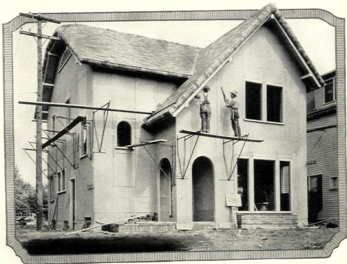
Residence in Indianapolis with Celotex sheathing as a stucco base. Maurice E. Thornton, Architect.
