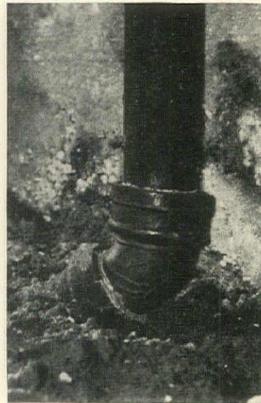
No clean-out here means that the plumber will have to take the pipe apart whenever stoppage occurs, involving considerable inconvenience and expense
