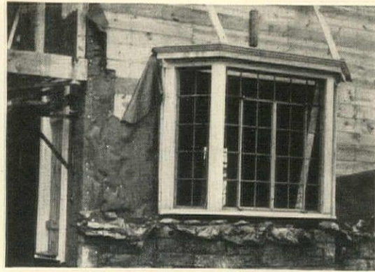
In contrast is the horizontal sheathing, the torn building paper and general unworkmanlike appearance of this new home, presaging future failures and repairs
