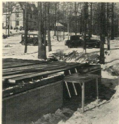
Another view of the same house, showing how the copper barrier is placed to include even the unbuilt brick chimney
