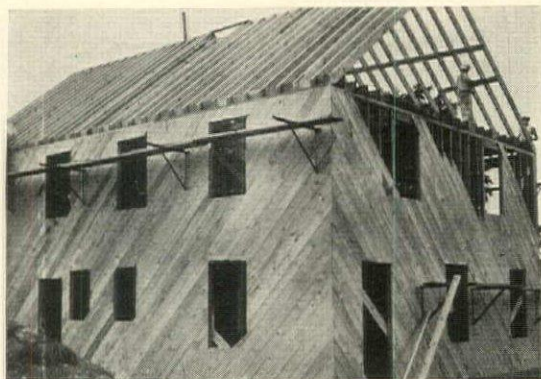
Diagonal sheathing not only covers, but adds rigidity to the entire structure, effectively bracing the house frame against wind pressures and other stresses
