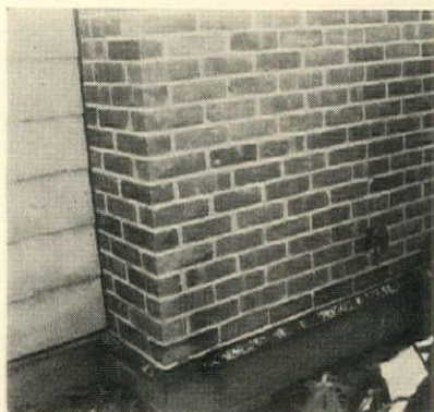
Here the chimney is completed, only a narrow ribbon of copper projecting. But no termite can get around or through it
