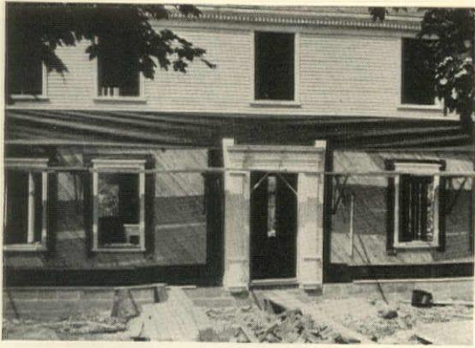
Careful workmanship in every detail makes the well-built house. Note diagonal sheathing, primed door and window frames, cleanly applied building paper
