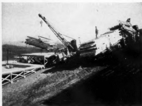
Parts of a prefabricated house are delivered at the site where they are quickly assembled. Improvements in this type of rapid construction are on the way.
