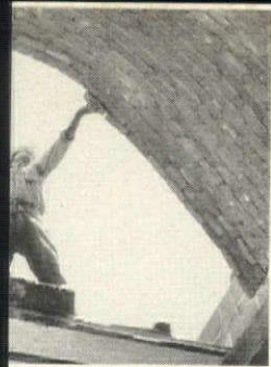
ew Mexican masons can build a bóveda. Mason follows the curve of his hat brim in coping the vault's contour.
