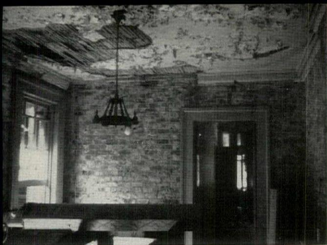
In dining room, cornice was broken, plaster almost gone.
