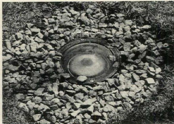
Quickly installed ground illumination: outdoor spotlight imbedded in pebbles. Water drains off into ground; light can be lifted out easily for any repairs.
