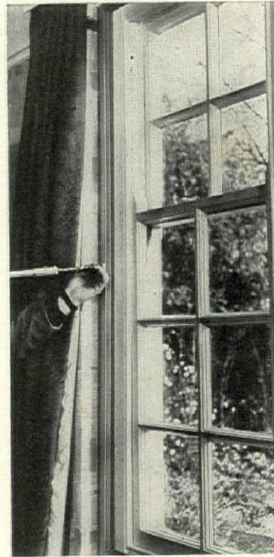
Fitting a custom-made window by Alpine, following sight line and applied direct to existing frame. More details from Alpine Everest Group, Alpine House, Honeypot Lane, London NW9
