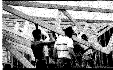
Erecting trusses was matter of only a few minutes and roof sheathing was done just as fast.
