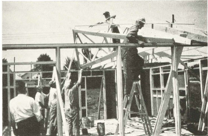
The 16 trusses used on this house weigh only 70 lbs. apiece, are easily handled. Light metal framing anchors are used to fasten trusses to wall plate. Nails can thus be loaded in shear.
