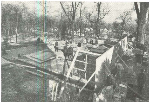
Cleared slab furnishes an ideal work surface for assembling wall sections. This house had two small furnaces installed above ceiling. Cost: $50 more than one large furnace.
