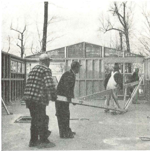
Four-man crew easily raises trusses to top plate. As soon as first few are up, the plywood roof sheathing can begin.
