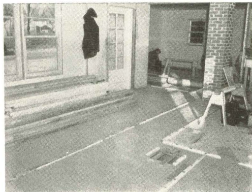
Flooring can be started at either end and sweep across an area uncluttered with a forest of studs.
