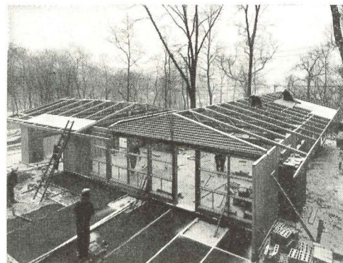
Plywood roof sheathing goes on fast with little cutting. Each sheet erected can be work platform for next.
