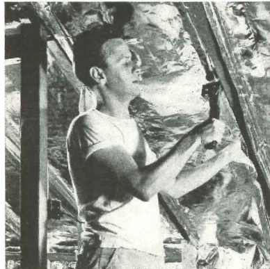
Designer staples aluminum foil insulation to nailing strips on beams to make room for recessing panels.
