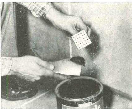
1. Adhesive is buttered onto anchor plate (below) which has protruding nail in center.
