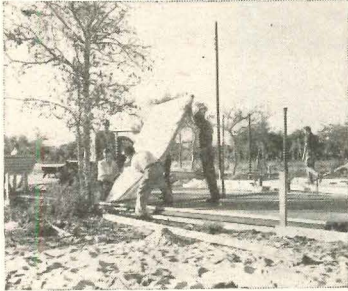
After honeycomb panels have been delivered, each is lined up on a 2' x 3' plate.
