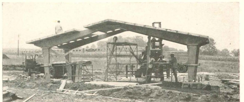
7. Roof planks were put on as soon as possible after each pair of bents went up. This picture was taken about two hours after first bent was installed.
