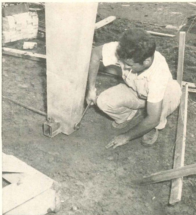
5. Footing connection includes built-in device to make bents plumb. Base of bent has 4" x 3" steel box to which reinforcing steel is welded. Box section projects on each side, has holes for anchor bolts. Bent is plumbed by adjustment of nuts over and under connection plate. Tie rod relieves bent of any outward thrust.
