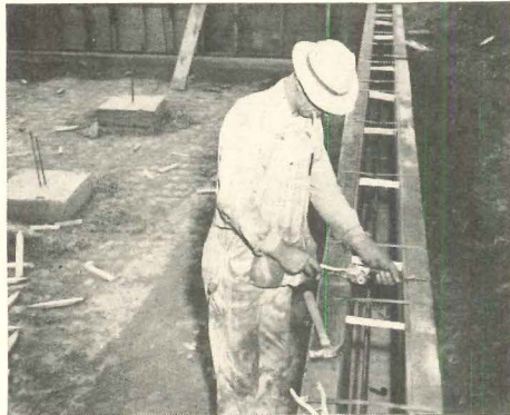
Steel straps , easily put on and cut off later, hold metal foundation forms together while concrete is poured. Wood spacers are removed and can be used again.
