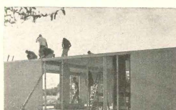
At day's end whole house is closed in—convincing evidence that prefabrication is a natural even for one-time structures.
