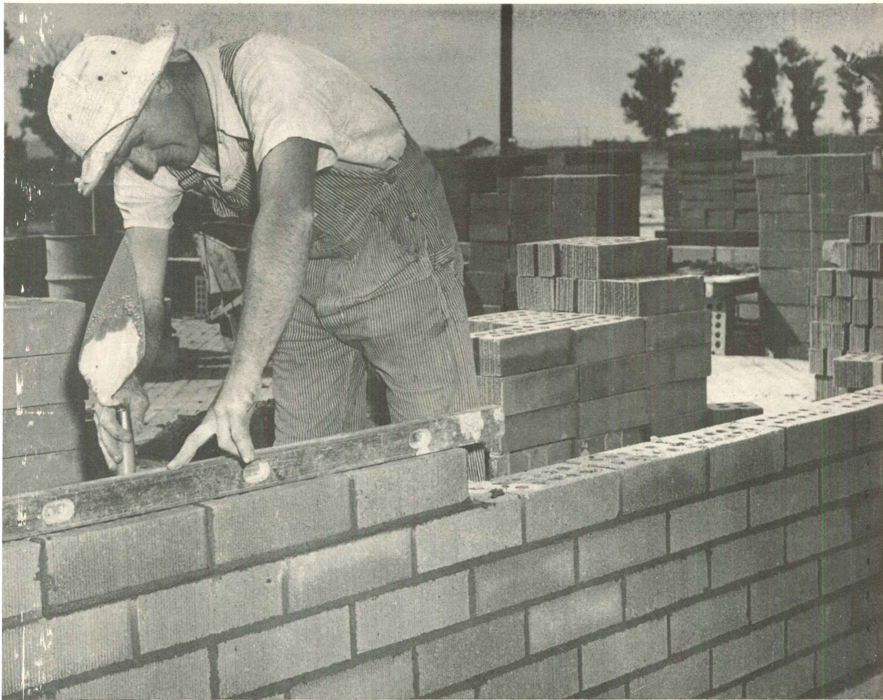
Seven men and four helpers put up walls in eight hours, use 2,200 jumbo bricks, 150 half bricks, 300 regular bricks for window sills. Big bricks do not tear masons' hands because workers pick bricks up before they are quite dry, placing fingers over edge, thumb in middle hole on one side. This smooths gripping edge. As experiment, Brockbank built some houses with regular-sized brick, found they cost $190 more. Bricks were developed and made by Interstate Brick Co.
