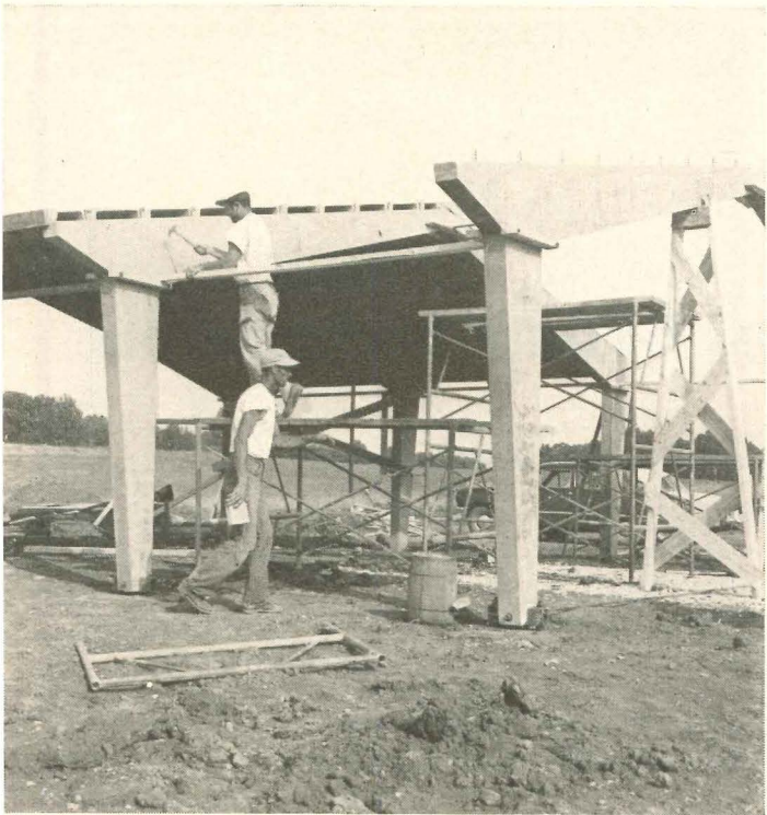
6. Temporary bracing supports bents as workmen here prepare to add more concrete roof slabs. Lateral stability is primarily obtained through the masonry walls put between bents later; transverse stability by the hinge action at each footing and where bents meet at ridge.
