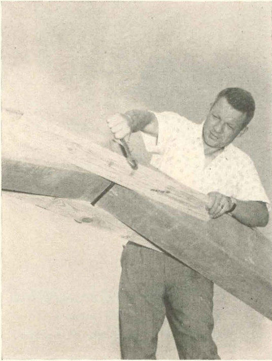
3. Bents are joined at ridge of house. Dowel pin drops through top of one bent into hole in a steel pin inserted through steel plates built into each bent.
