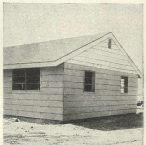
6 Another Duraply home finished! Savings on material and labor costs—as well as savings on painting costs and time—have given this builder an extra profit margin. Plain-panel Duraply is also finding wide use for soffits and gable ends.
