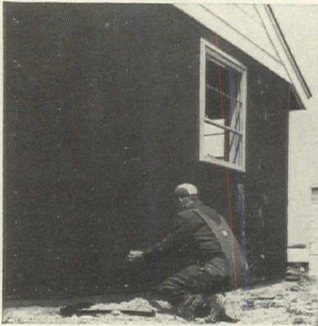
1 Workman checks level before installing first course. Duraply is exterior grade plywood with a permanent "CreZon" overlay bonded to its surface. "CreZon" (phenolic resins and cellulose fibers) is strong, weatherproof, supersmooth.
