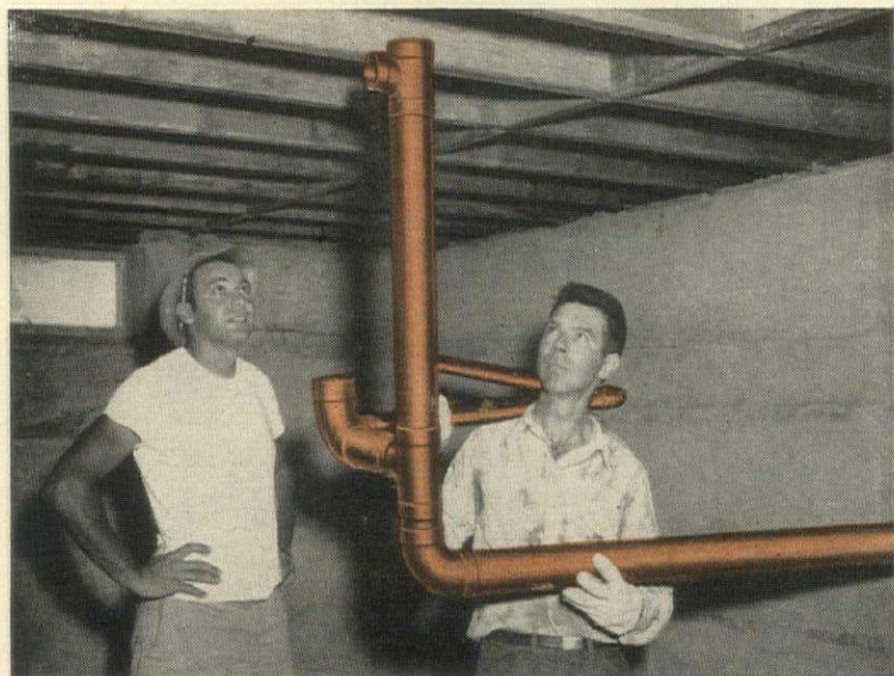
Lightweight for easy, fast handling. This preassembled section comprising about 13 feet of copper tube and 5 solder-joint fittings weighs only 35 pounds, is easily handled by one man.
