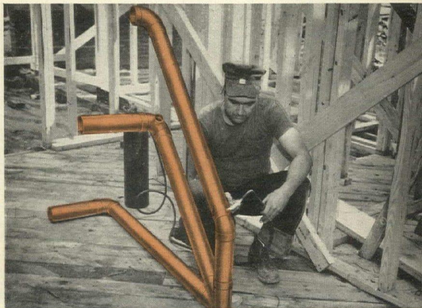
Prefabrication speeds construction. Sections like this can be preassembled out in the open or at the shop where men can work easier and faster—no lost time waiting for construction.
