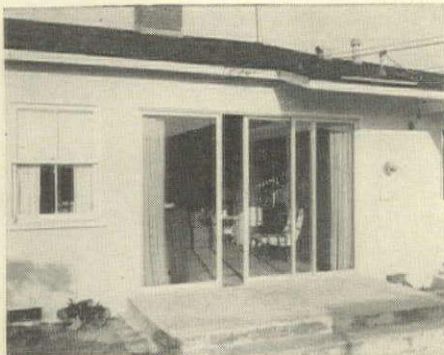
AFTER: First stage. When complete, service conductors will be relocated and roof extended to shelter the new terrace.
