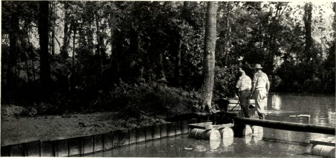
SHEET STEEL PILING forms bulkhead for each new bay-side lot. Piling costs $30 a running foot. Since lots average 100' wide, this raises their cost $3,000. So bay side lots sell for as high as $12,000, while lots on lake side (without piling) are valued at $6,000 to $8,000.
