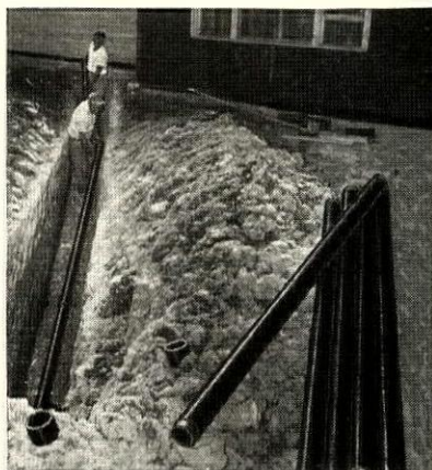
Sewer installation at a project home, by N. J. Rodrigue, Plumbing Contractor, Houma, La. Permaline comes in 5, 8, and 10-foot lengths. Diameters 2, 3, 4, 5, 6, and 8 inches. Full line of fittings, adapters.
