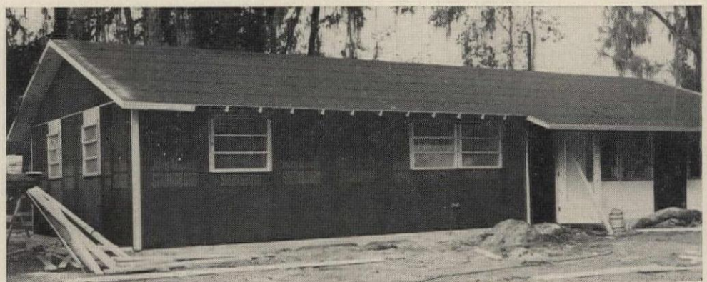
ALL CLOSED IN by 4:30 pm, the house is ready for the plumber and carpenters to work inside the next day. Dyches modeled his building schedule
