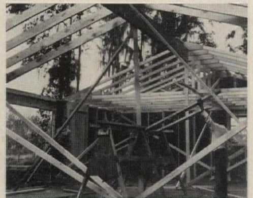
SLOPING CEILING components (used over the living room) are set atop plywood box ridge beam resting on posts between trusses.
