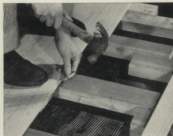
Over concrete, install Strip Oak Flooring this low-cost way... on screeds imbedded in mastic.
