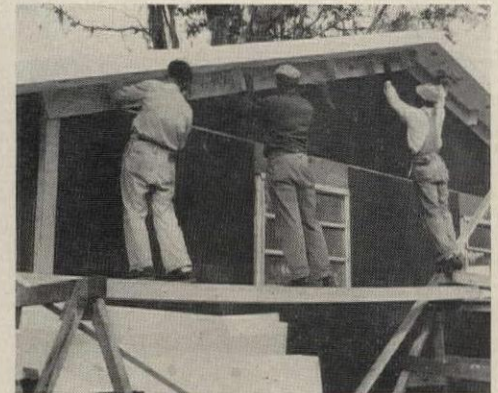
PRE-BUILT FRIEZE board blocking is nailed to the underside of the gable end before the house is brick veneered.
