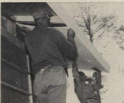
SOFFIT , fitted into groove of fascia, also bears against a metal angle nailed to the heel block on trusses, to prevent buckling.
