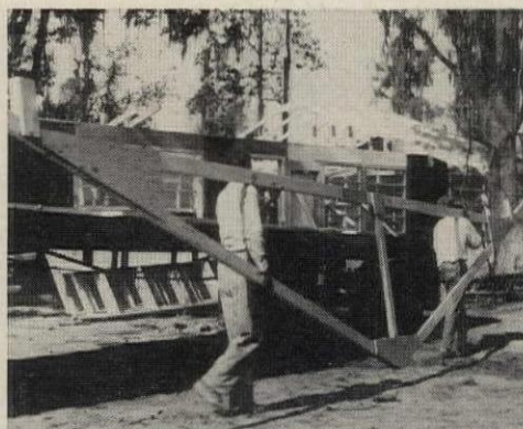
TRUSSES go up as soon as all wall panels have been erected, generally before noon. Here, 4-in-12 king-post trusses are used.
