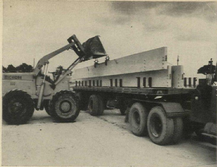
GRADE BEAM is lifted from truck by special tongs on loader bucket.
