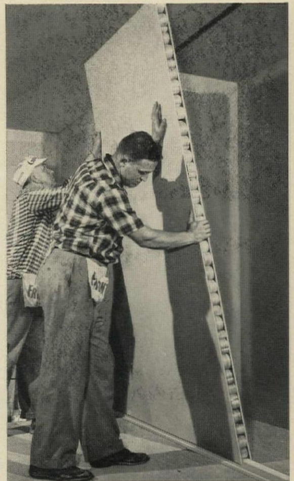
IN PLACE FAST. Two men can easily put panels in place. Top is secured by nailing through corner bead into wood spline in panel.
