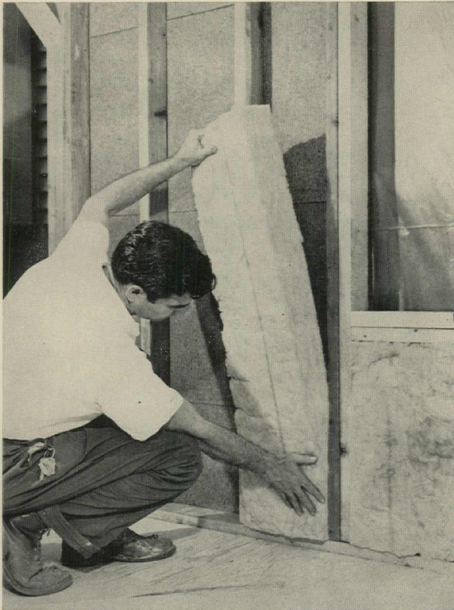
FRICTION-FIT BATTS are easily handled, easily cut. Installer can put them in place almost as fast as his helper can hand them to him. Snug fit assures no leaks. (No. 1)
