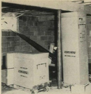
PACKAGED PARTS —boiler, water heater, and supply lines—are delivered to the spot where they will be installed.
