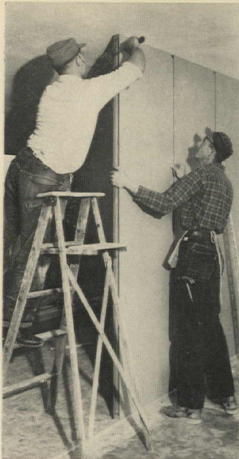
PARTITION PANEL sits on floor runner, is nailed directly to ceiling through top rail. Wide joints between panels accentuate panelized look.
