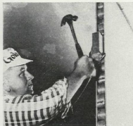
ANY 2X BLOCK can act as spline between panels. Door buck is 2x2 set between faces.
