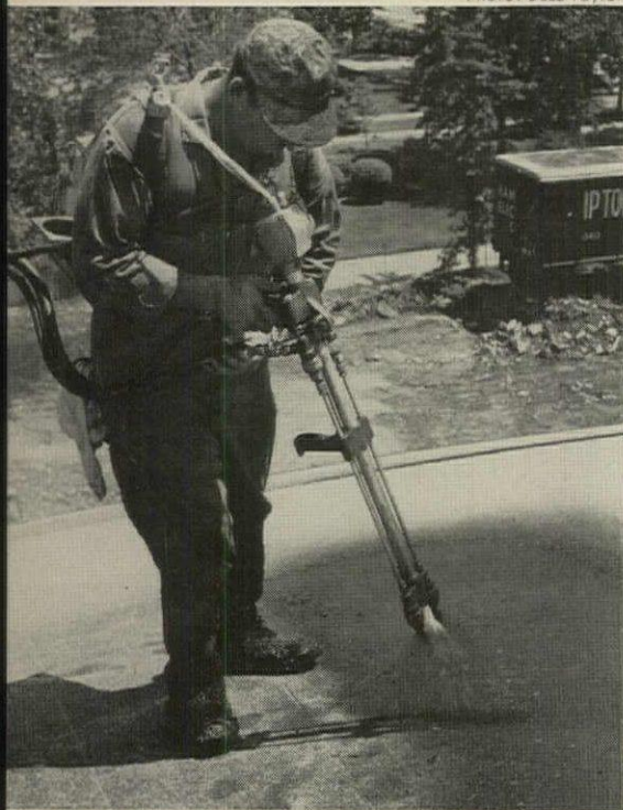
MULTI-NOZZLE GUN sprays chopped glass, asphalt, resin, curing agents, and other materials to make a one-coat roof.
