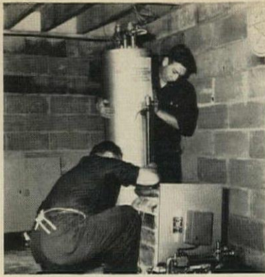
HEATING UNITS come in two big packages, go together with only two joints, freeing men to work on baseboards.
