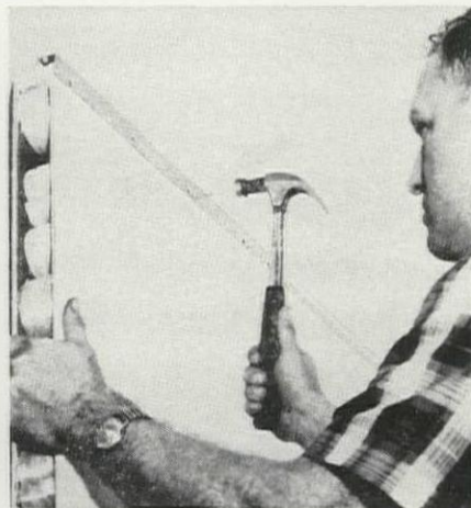
CORNER BEAD on ceiling acts as hanger. Panel is jacked in place, nailed head and foot.
