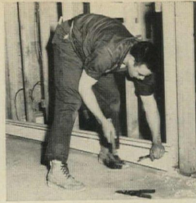
BASEBOARDS are quickly nailed to studs. They are cut to size before delivery, and shipped in color coded cartons.
