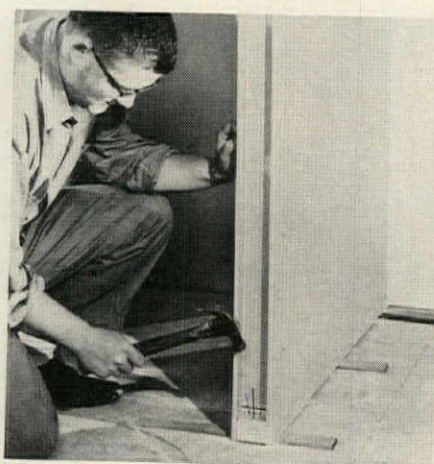
2 Panel is jammed against ceiling by driving shims under bottom edge. It is end- and toe-nailed to floor through the bottom plate.
