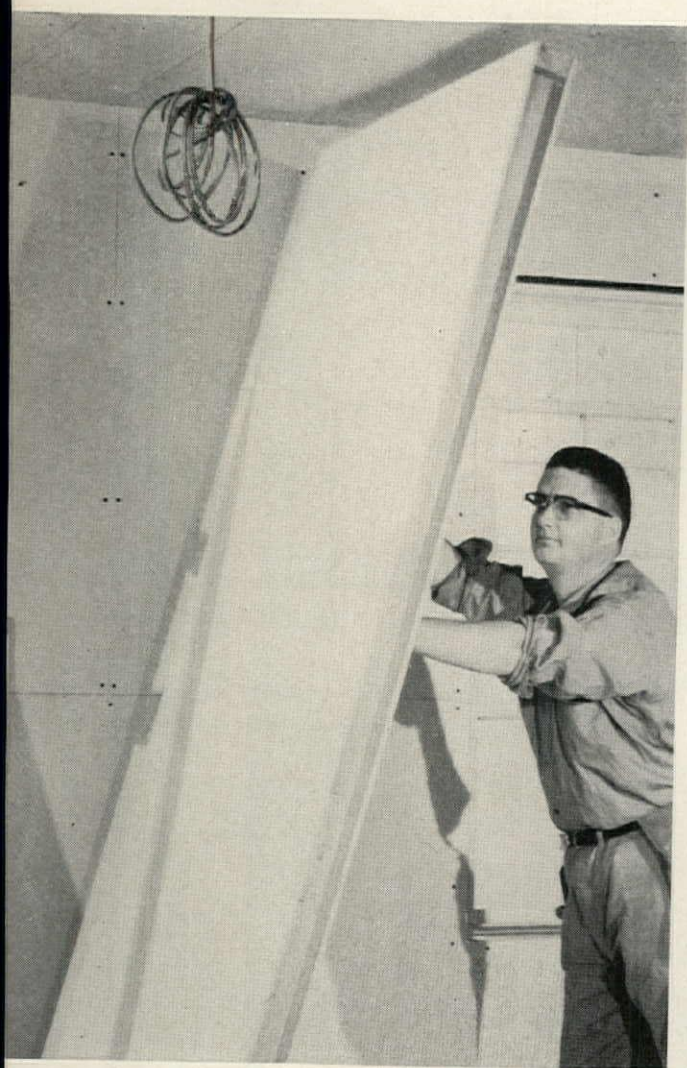
1 Partition is started by nailing cleat to outside wall, then tilting up panel and slipping its recessed edge over the cleat.
