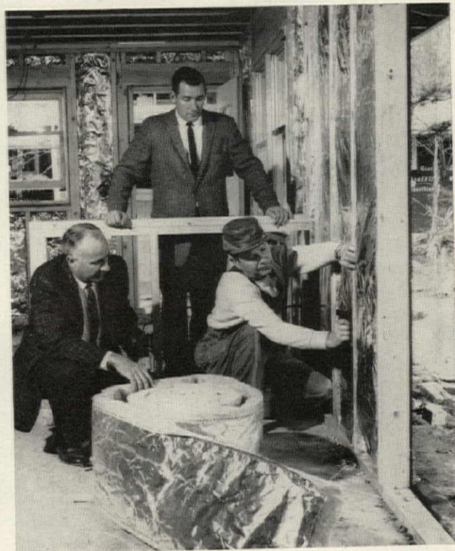
PROPER INSULATION builds-in economy and comfort. Hobart Smith uses 2" insulation in floors, 3" in walls, and 6" overhead, conforming to the All-Weather Comfort Standard.
