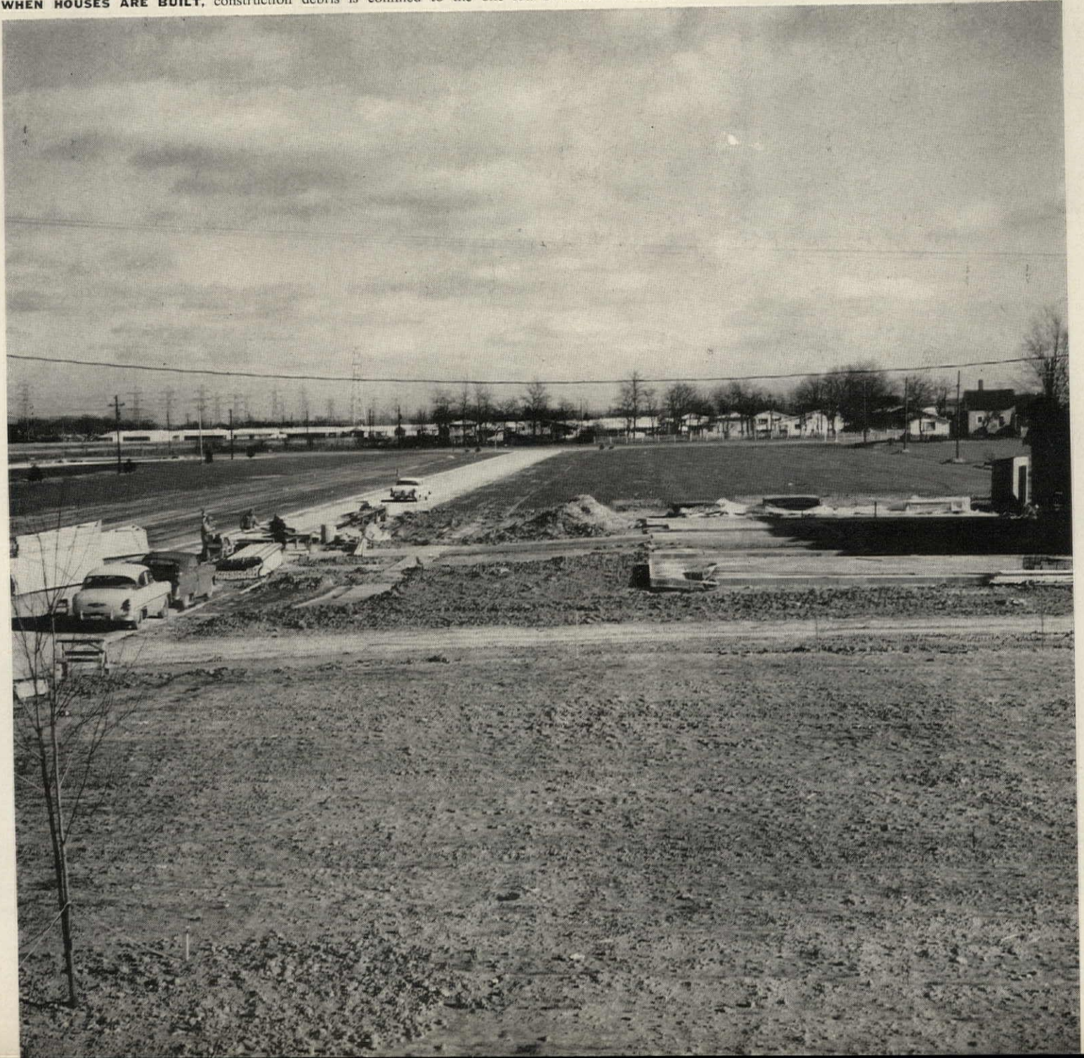
WHEN HOUSES ARE BUILT, construction debris is confined to the one lot. Schmitt's 7"-thick concrete streets can carry heavy trucks without cracking.
