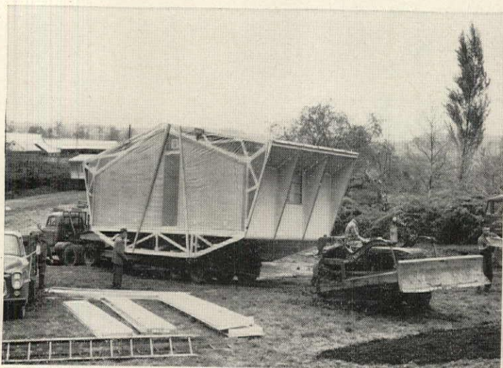
1 Tractor helps trailer back up slope to put first section in position for crane. Difficult sites would call for a tractor tow like this.
