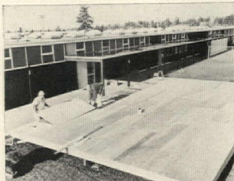
FIRST DAY: Conventionally built unit's plywood floor deck goes down in 35 minutes. Floor framing members 4' oc support 5/8" thick t&g deck.
