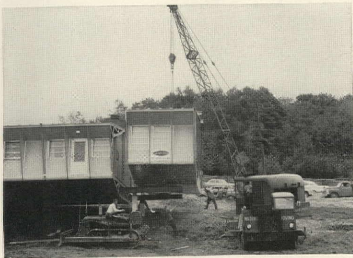
7 Last section is swung into place, and major part of field work is done. Power is now on, and cables to tie sections together are being placed.
