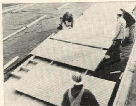
THIRD DAY: 2x4 wall framing assembled on floor deck is sided with textured plywood. Black polyethylene sheet protects deck from weather.
