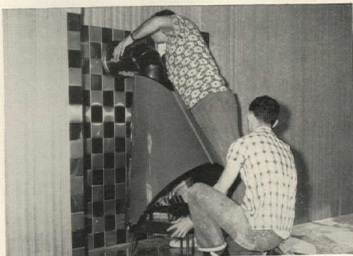
11 Fireplace is finishing touch. Steel tiles reflect heat, and flue heat exchanger ties into central system to boost warm-air supply.
