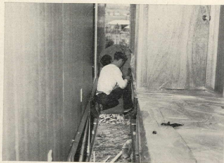
6 Gaskets to keep weather out when house expands and contracts are placed around trusses before one section is jacked against another.
