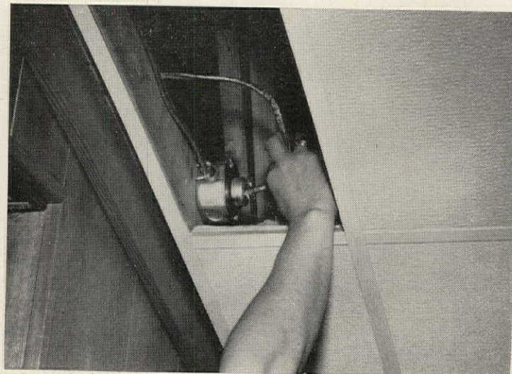
10 Power hookup between sections is made with a twist lock plug. Underground service in conduit enters belly of mechanical section.
