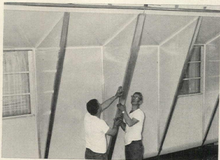
9 Cap strips of aluminum cover gasketed joints between sections after ten cable ties have been tensioned to 1,600 lb apiece.
