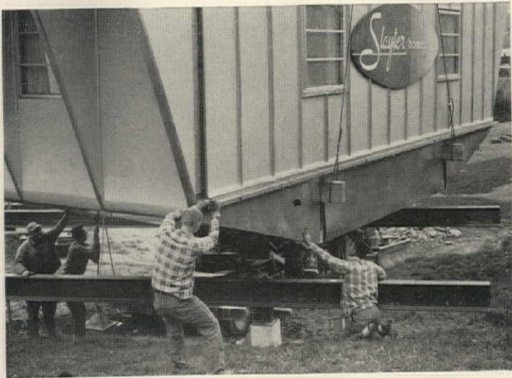
3 Positioning first unit must be exact so next one can be jacked against it. Lifting beams, two 2x8s, are cut off flush, become part of house.
