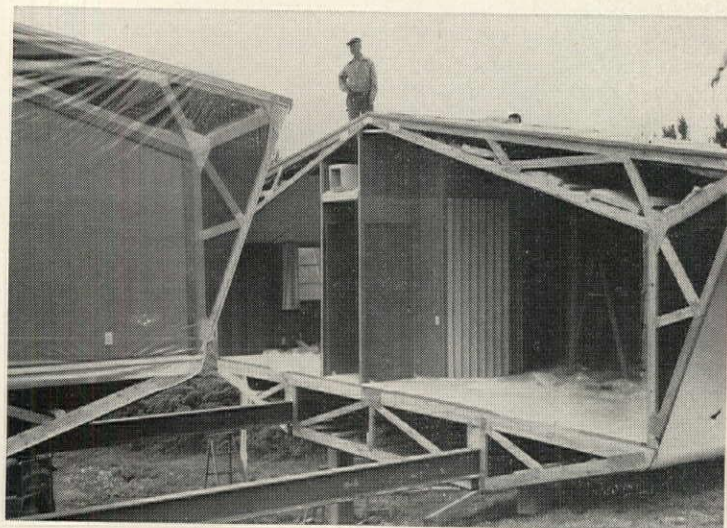
5 Ready for joining, first unit has had lifting beams cut off flush and polyethylene stripped off. Air supply duct is over bedroom hallway.
