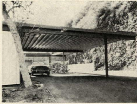
Carport shows basic post, beam, and decking construction. Note steepness of hill at right.
