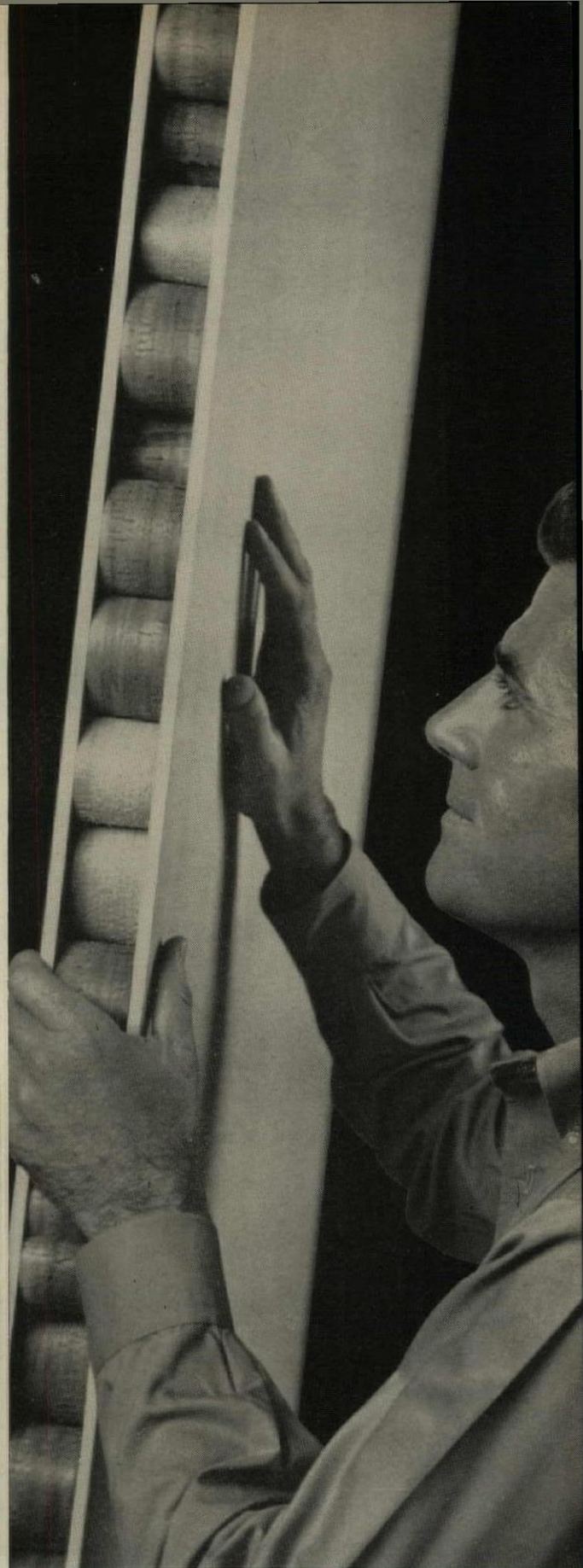
Large 4' x 8' panels go up quickly and easily, with less nailing and fastening, and reduced erection time.
