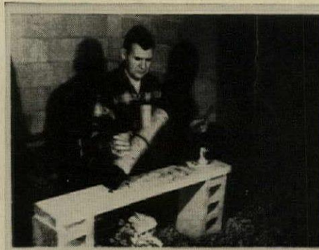
1 Plumber begins on-the-job joining of ABS DWV fittings and short lengths of pipe for the assembly which will be installed in the basement. Cutting to length, brushing solvent cement on both pipe and fittings and making the joint is accomplished in a few minutes.
