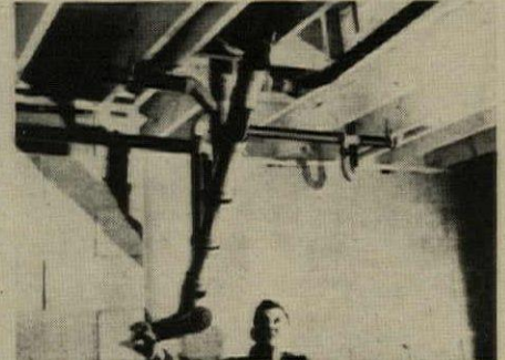
4 Completed basement installation is given final check. At this point, two men had assembled and installed the plumbing tree, and are ready to start work on first floor.
