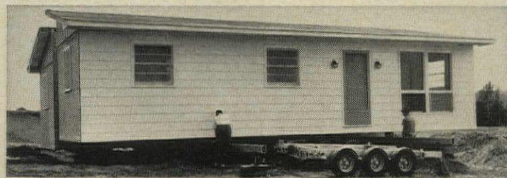
MOVING INTO POSITION , section has been lowered to rest on rollers on the steel beams. It is then pushed into place against the other half. Next, the section is raised on the jacks, beams are removed, and the section lowered to exact position. System takes about 12 man-hours, eliminates crane.
