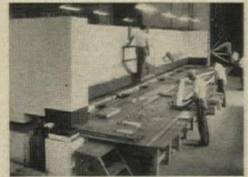
TRUSS PRESS at Pease is a mass of concrete operated hydraulically by a 3-hp. motor. Time per truss: 10 man-minutes.
