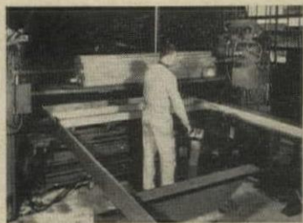
FRAME NAILER at Arbor Homes, operated by one man, nails plates and studs for 2,500 feet of wall per 8-hour shift.
