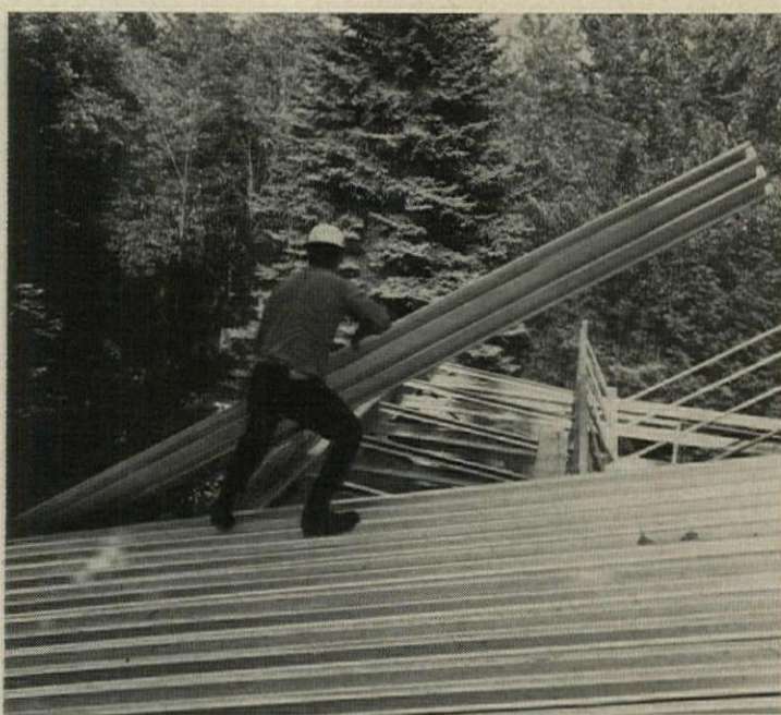
ARMCO ROOF PANELS are ridged pans 24" wide and 2" deep, rest on a complicated framing system of lateral and longitudinal trusses. The pans themselves form the roof surface. The prototype house being erected above and at left was designed by Architect Carl Koch.
