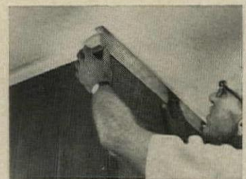
ANGLE of galvanized steel is nailed to top of wall and underside of roof to anchor roof to cedar-plywood wall surface.
