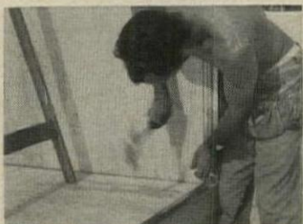
TOE NAILING fastens wall panels to floor. Vertical panel joints are made by toenailing each panel edge to a spline.
