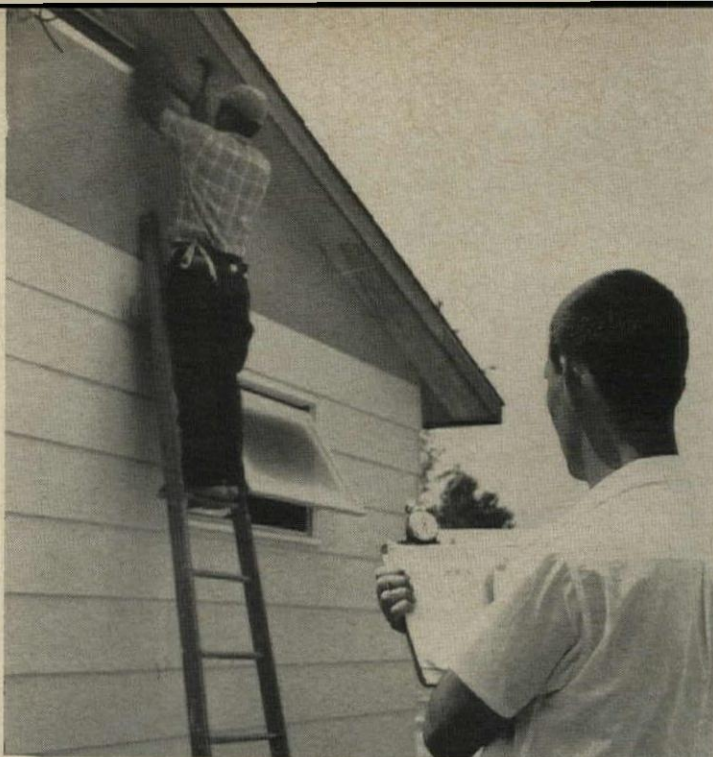
TIME-AND-MOTION STUDIES helped Project TAMAP analyze methods of efficient Builder Bob Schmitt, revealed many ways to make him even more efficient, and showed how manufacturers could improve their products to contribute to easier, lower-cost use by builders.
