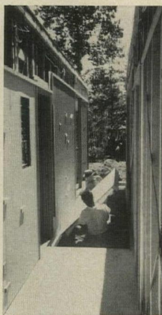
FLOOR PANELS are dropped into center of Boester model after side sections have been set on foundation and piers.
