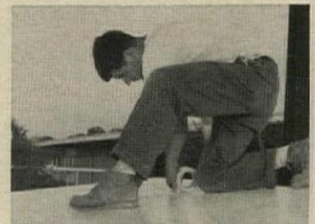
TAPE is hand applied to plastic surfaced roof panels to seal the joints — finishing the job. No further roof finish is necessary.
