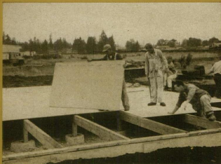
1. Foundation was poured the day before. Plywood floor on this model is 2·4·1, the 1½-in.-thick combination subfloor-underlayment, with supports on 4-ft. centers.
