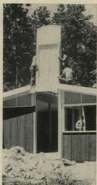
FRONT-DOOR PANEL fits so precisely into center section it has to be dropped plumb into framed slots on the side sections.
