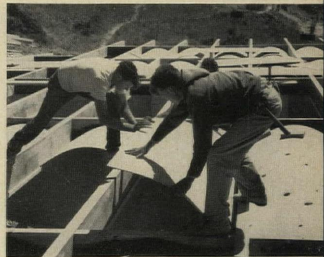
Curved plywood soffits conceal pipes, wiring and insulation under the floor. Pre-painted panels of 1/4" EXT-DFPA plywood were sprung between 4x12 framing. This is an easy way to conceal the clutter under a hillside house. The heating and cooling system are also out of sight, in the attic plenum.
