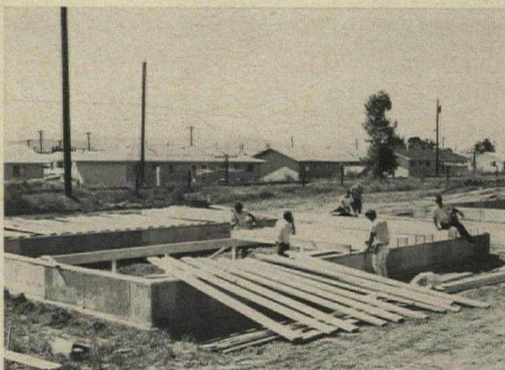
FLOOR-SYSTEM RESEARCH evaluated five types of floor deck installed under identical conditions. Results: Cheapest system was 2 x 10 joists laid on 2' centers, fastest was LuReCo's "Insta-Floor"; but differences among all five systems were small. Complete results will be announced soon.
