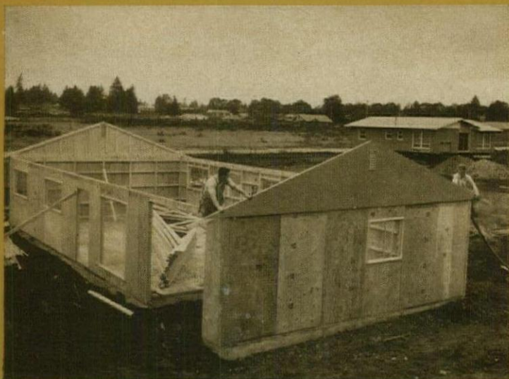
4. By 10:30 (2½ hours after the start of work) the crew is ready to lift prefabbed gable ends into position. Almost at the same time, they begin installing trusses which are waiting inside on the floor.
