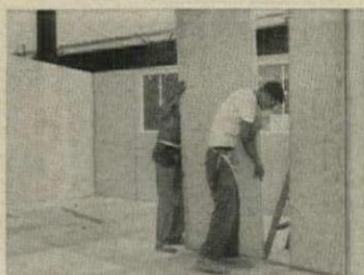
WALL PANELS have a kerf in their bottom edge so they can be easily positioned on galvanized tees nailed to the floor.
