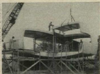
MONSANTO PLASTIC HOUSE was a spectacular demonstration of the structural possibilities of reinforced polyester plastic.
