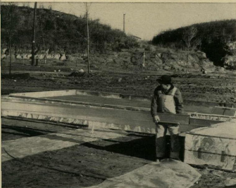
STEEL FLOOR BEAMS are set in hangers on beam. Plastic vapor barrier is set under jacks, then folded back so workmen will not damage it.
