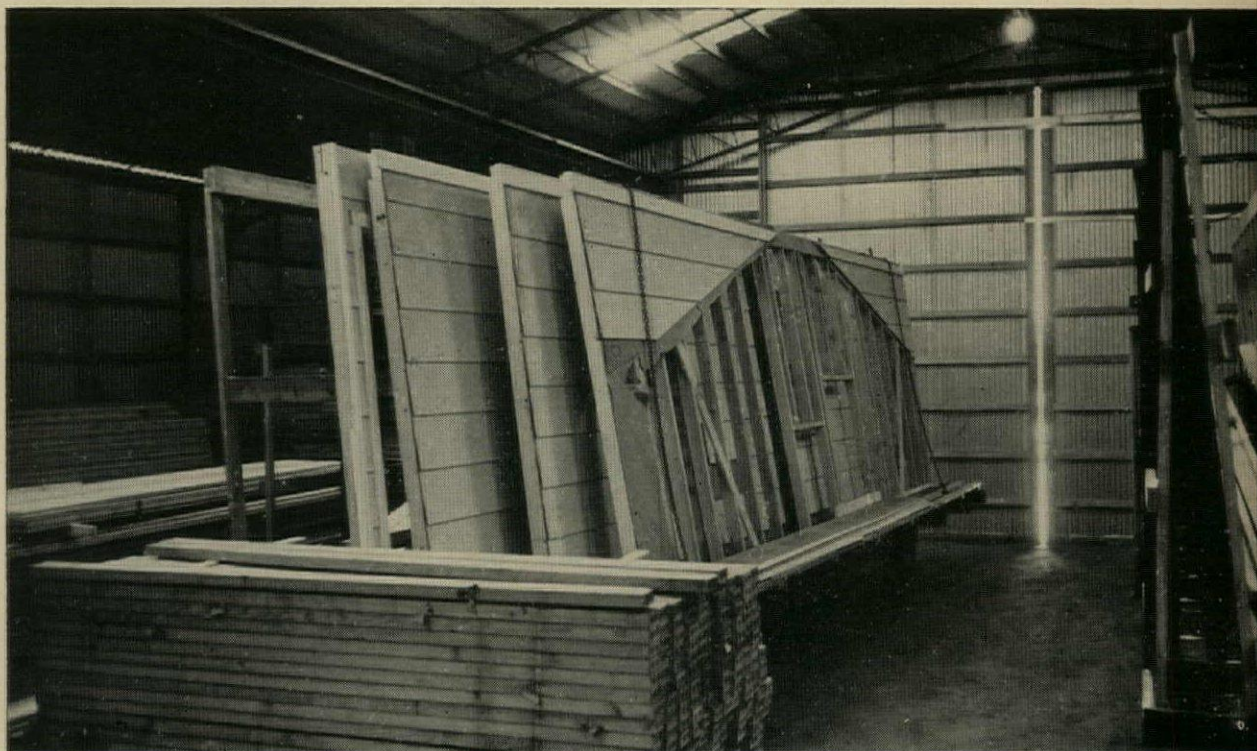
COMPLETED PANELS are stored on trailer ready to be erected. Open panel on side will abut the garage ell of the house. When the weather breaks, the house can be hauled to its lot in minutes.
