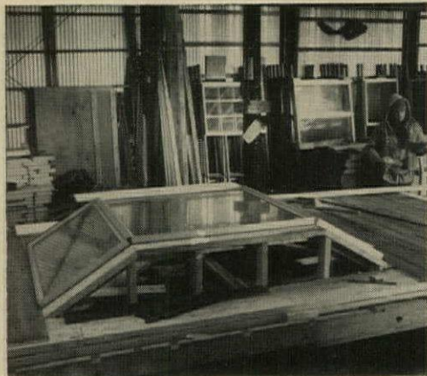
BAY WINDOW is framed, glazed and trimmed right on the wall panel. Since window protrudes, panel will be the last one loaded on the trailer.
