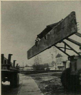
PRESTRESSED GRADE BEAM is lifted off truck by front-end loader with "ice-tongs" on bucket.
