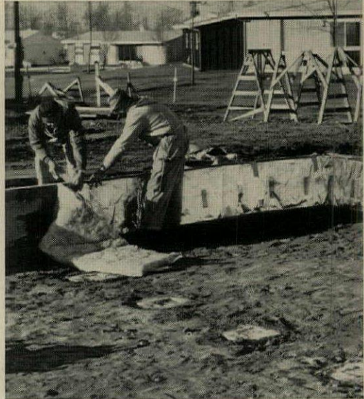
PERIMETER INSULATION is fastened to beam with pressure-sensitive tape (right). Shallow concrete pads, bottom, provide bearing for steel joists.
