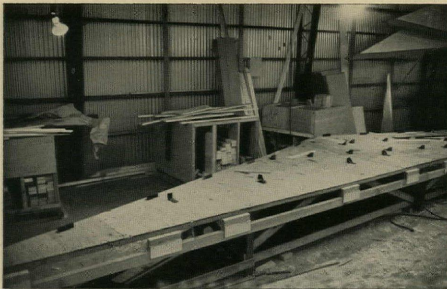
GABLE-END JIG can be adjusted for different widths and pitches. Metal stops are set in holes which are color-coded for various sizes. Box (rear) contains shorts cut from scrap for gable studs.
