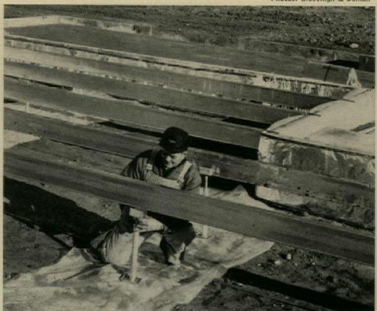
SCREW JACKS are placed under steel beams for intermediate support. They permit use of same depth beam to span any width of the house.
