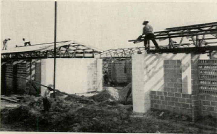
LOCAL WORKERS fabricate roof trusses on site, hoist them onto the walls of hollow concrete blocks. The floors are concrete tiles on compacted soil.
