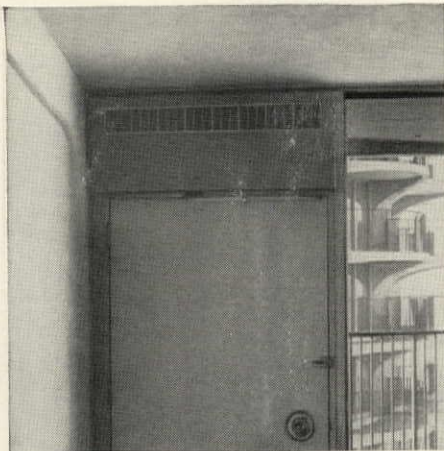
Again demonstrating its flexibility, a Zoneline unit has been installed above a door in a typical Marina City apartment.
