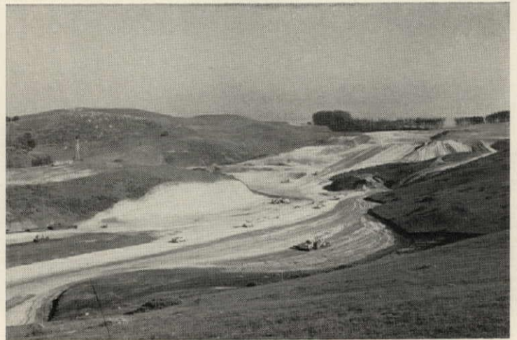
ROLLING HILLS call for careful layout of haul roads to give loaded scrapers downhill runs.
