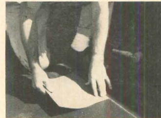
3. First tile is laid on point marked at center of job layout.
