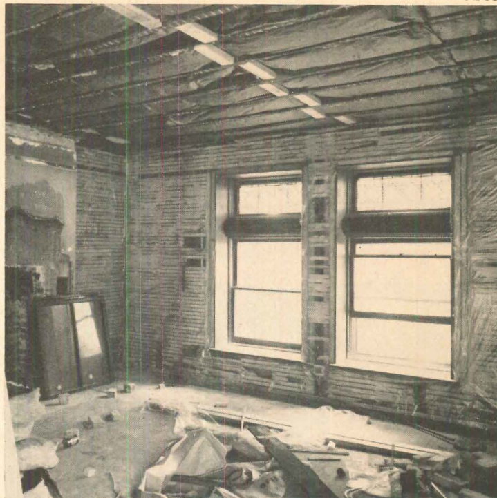
METHODICAL JOB-STRIPPING gets rid of unsound plaster, but old wood lath is removed only when new insulation is necessary, as in ceiling of top floor apartment, above. Unusual old windows are carefully saved.
