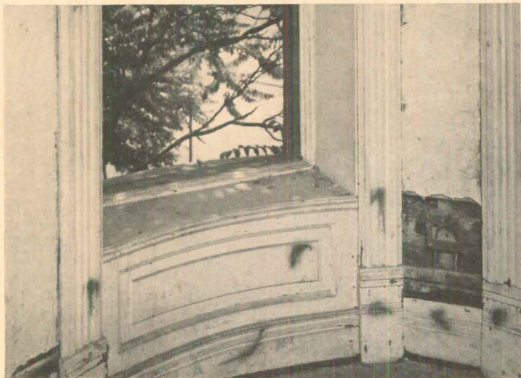
PRE-MARKED OLD TRIM —it's squirted with paint-spray can—tells workmen how to treat it. Different colors mean 1) leave in place 2) remove for use elsewhere in house, 3) save for warehouse stock, 4) discard.
