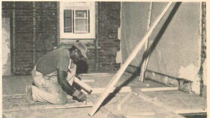
ALL-NEW PARTITION LAYOUT goes exactly like new construction. Old plaster on party wall, right, is covered by new plaster after metal lath is attached by 2" shingle nails driven through old plaster into brick wall.
