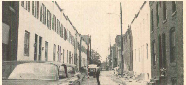
TIGHT LINEUP of narrow rowhouses is ideal for production-line work. Remodeler's ten-man crew works on 20 houses at once, which keeps subcontractors busy with no more than one trade in a house at a time.
