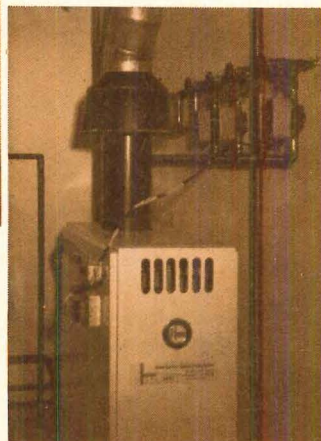
and zoned hydronic heating, of course.
