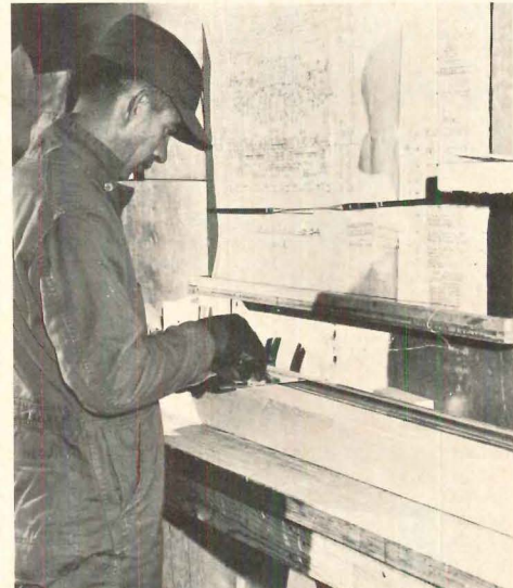
LAYOUT of wall panels is done by carpenter marking stud positions on top and bottom plates.
