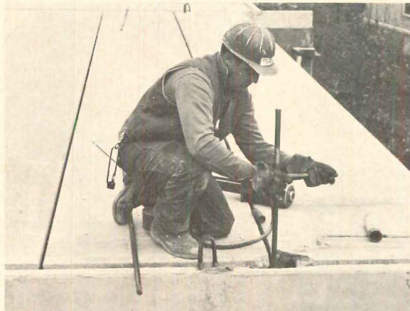
4. ROD TENSIONING , done floor to floor by hydraulic jacks, locks wall panel to walls and floor planks beneath.
