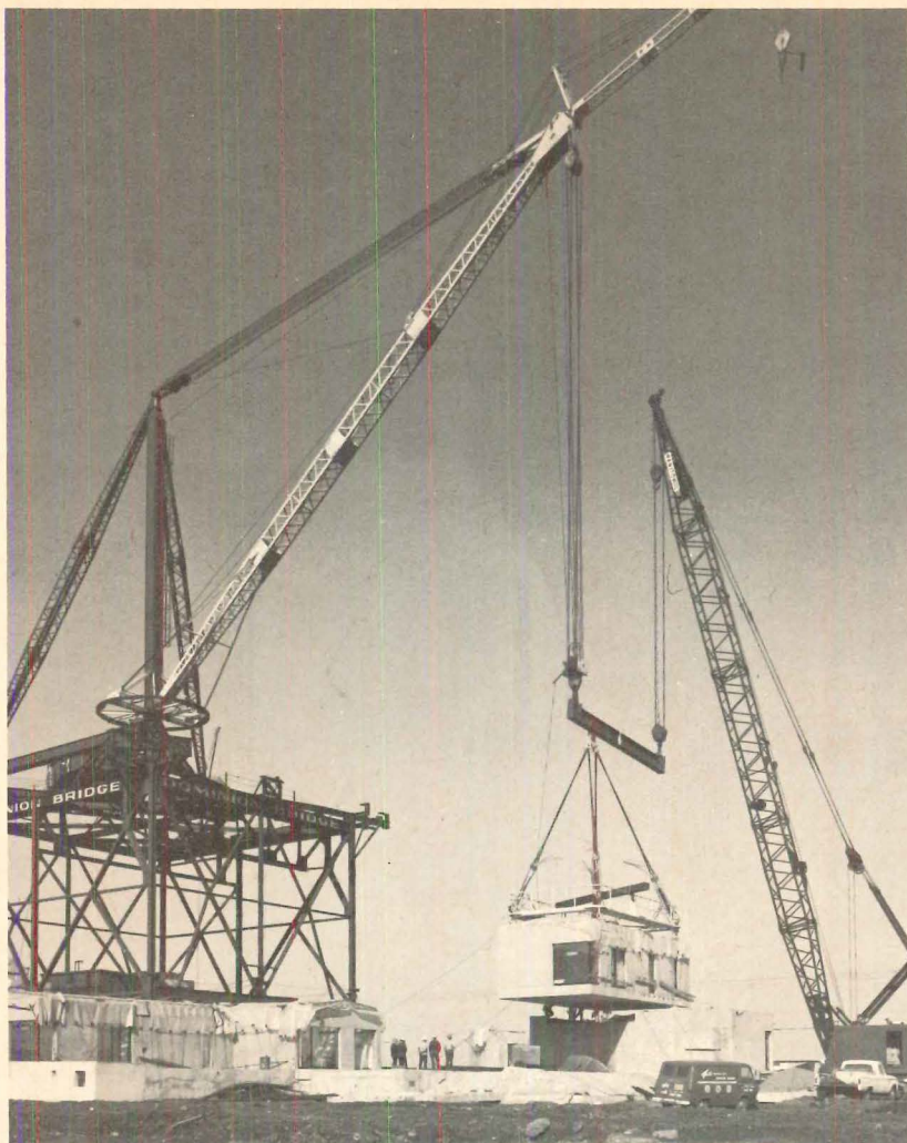
DERRICK AND CRANE hoist one of Habitat's 90-ton modular boxes (17½'x38½'x 10') during early construction. Interior finishes were applied before boxes were placed.
