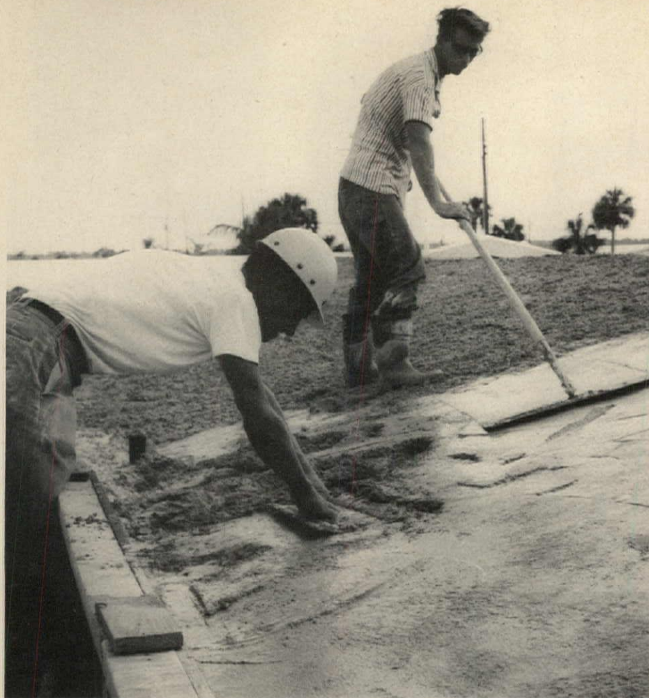
POURED ROOF DECK —with poured trusses underneath—is hand-floated prior to power floating (far right). Finished surface is painted with plastic and incorporates a drainage system.
