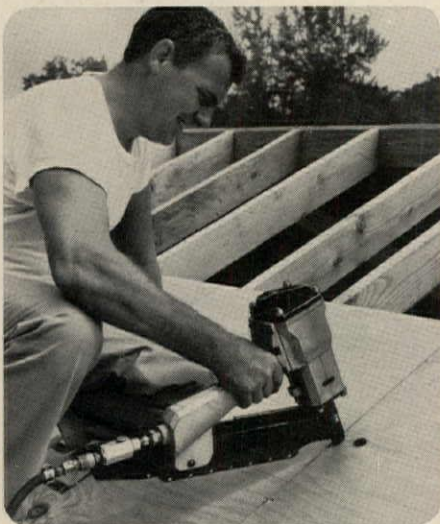
5. Plywood roof deck (or subflooring) is quickly installed with a CN-137 Nailer.
