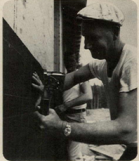
4. Building papers and moisture barriers are securely tacked with a Hammer Tacker.
