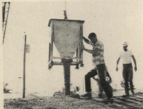
3,000-PSI CONCRETE of 5"-slump consistency is hoisted by crane and half-yard bucket.
