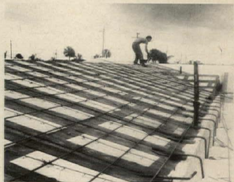
REINFORCING STEEL interlaces roof deck and ties bottom chord of trusses to bond beam.
