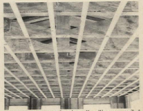
FURRING STRIPS for drywall ceiling are nailed to 1x4s cast into bottom truss chords.
