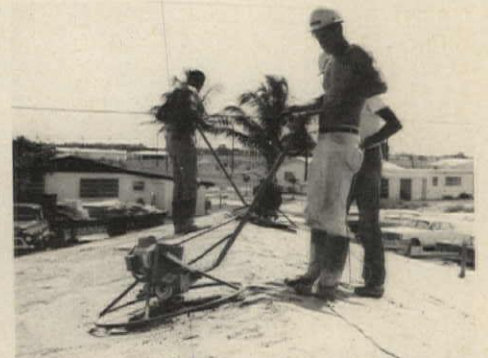
POWER FLOATS apply finished surface after concrete has been leveled and hand-floated.
