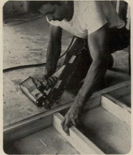
1. Wall assemblies are fast with a CN-137 Nailer driving coated 16d sinkers.
