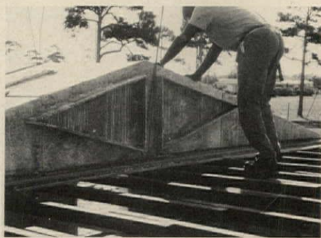
TRIANGULAR SPACERS , set on cleats in the truss forms, make voids for ducts and wiring.
