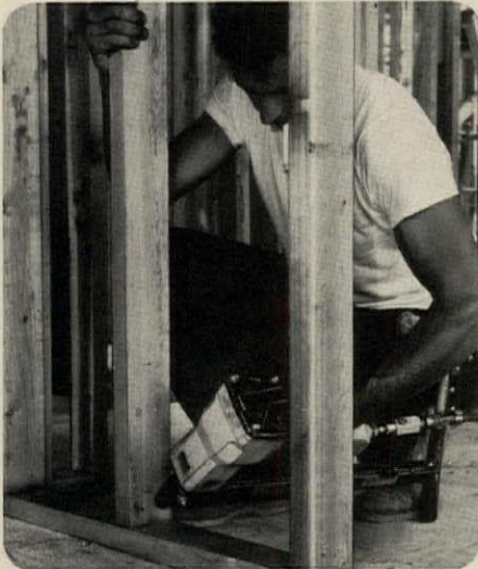
2. Toe nailing is easy the Duo-Fast way ... even working in overhead positions.
