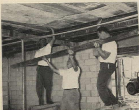
FORM REMOVAL is easy: When the steel channels are slipped out, forms fall to the floor.
