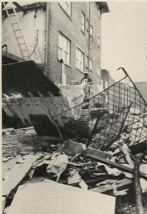
SLUM APARTMENTS in Cleveland involve heavy stripping and cleaning work. Rehab costs—while
