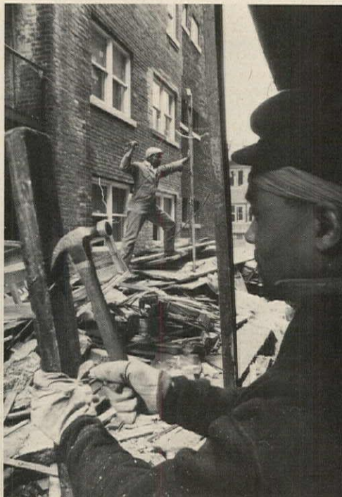
considerably less than total clearance plus new construction—range from $10 to $15 a sq. ft.
