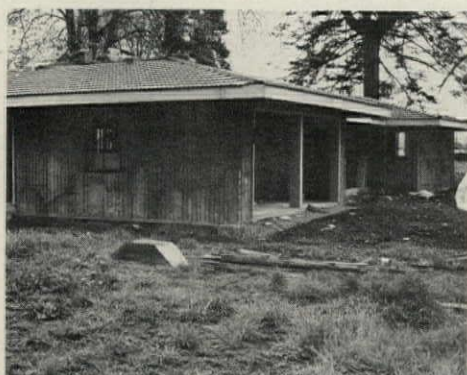
UNFINISHED HOUSE has concrete walls poured. Steel mesh is exposed to receive stucco finish.
