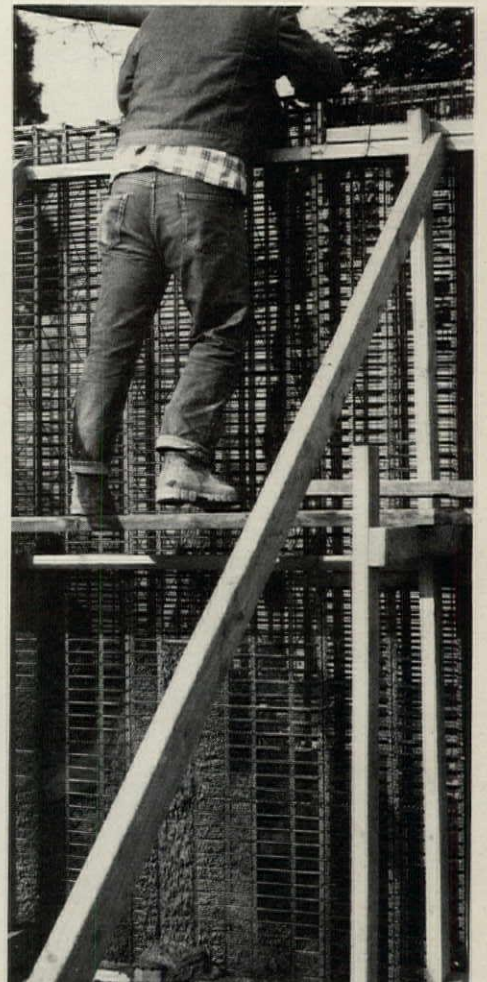
POURED CONCRETE oozes through steel mesh, is trowel smooth to cover steel. Stiffer mix oozes less, lets mesh act as lath for finish.
