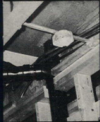
accommodate even large duct work.
