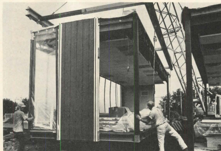
Modular classroom takes shape at PepsiCo Building Systems plant in Florida. Wood sheathing will cover a steel frame. Units weigh nine tons.
