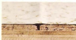
Regular flooring can crack or ridge.
