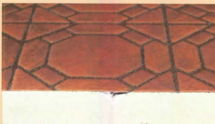
Tredway bridges subfloor problems.
