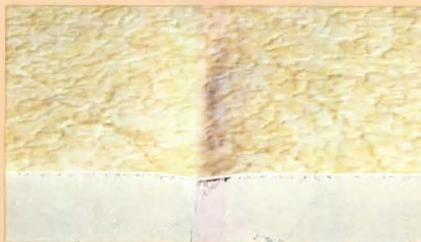
Conventional floors can telegraph subfloor problems.
