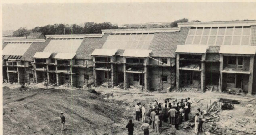
Denmark's zero-energy home, built to prove that a detached dwelling can generate virtually all of its own energy, even in a harsh climate; and solar-heat apartments being constructed for low-income families in Skive, which is known as the Danes' Energy City.
