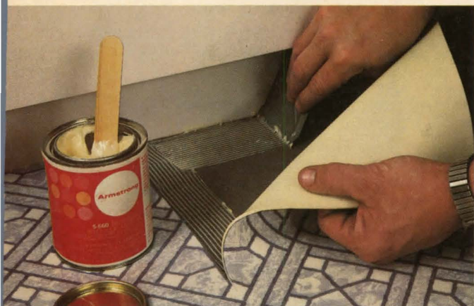
When installing under toe kicks or over concrete, all that is needed is a single band of trowelable adhesive.
